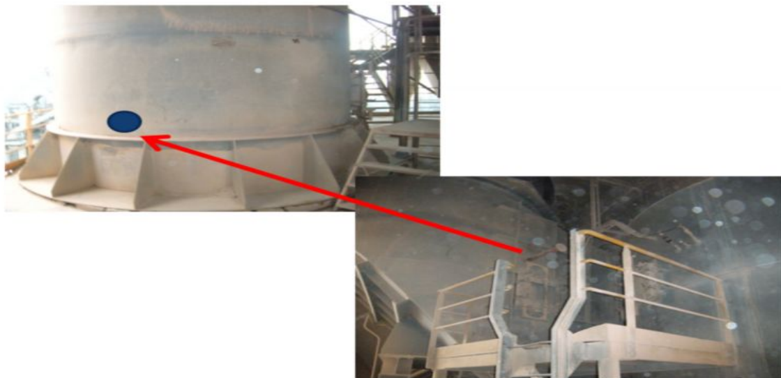
Figure 3.23 : Gaine gaz entrée cyclone 4
